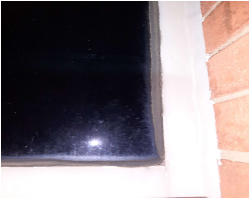
Photograph No. 4 – Black exterior window glazing contains asbestos.
