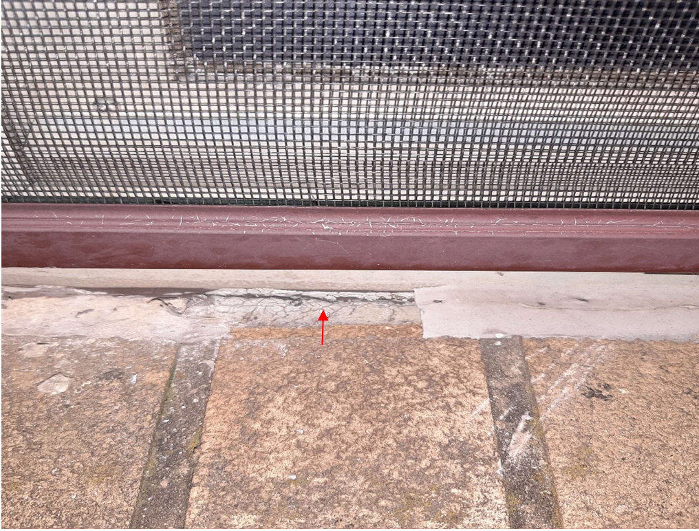
Photograph No. 3 – Exterior light gray sealant on windows (under light gray silicon sealant) contains asbestos.
