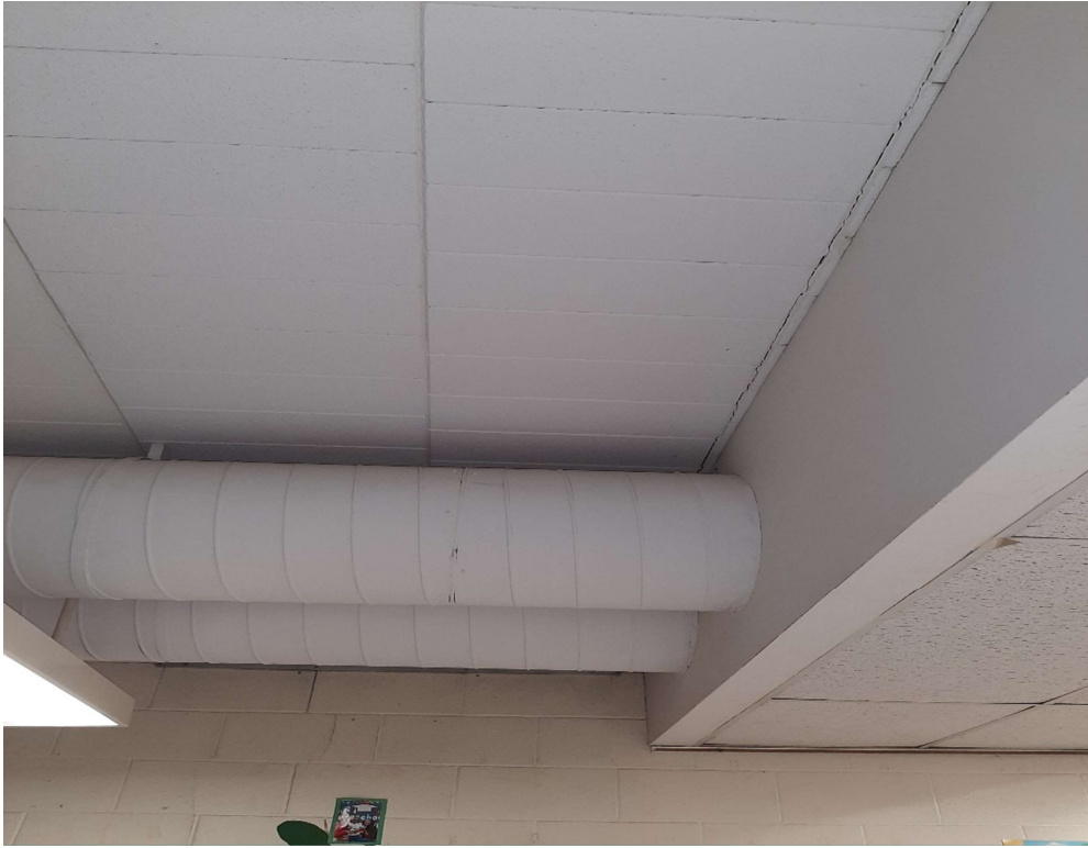
Photograph No. 7 – Drywall joint compound contains asbestos.
