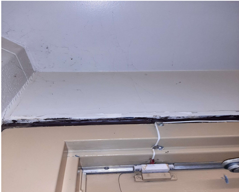
Photograph No. 6 – Drywall joint compound contains asbestos.
