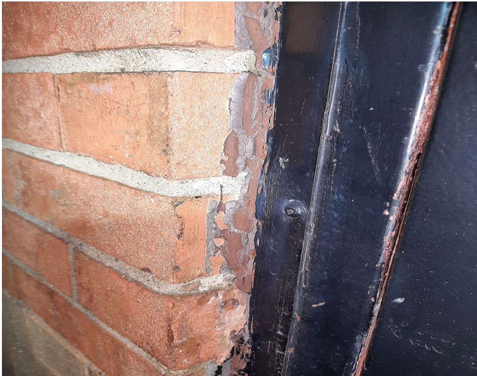
Photograph No. 2 – Exterior brown sealant contains asbestos.
