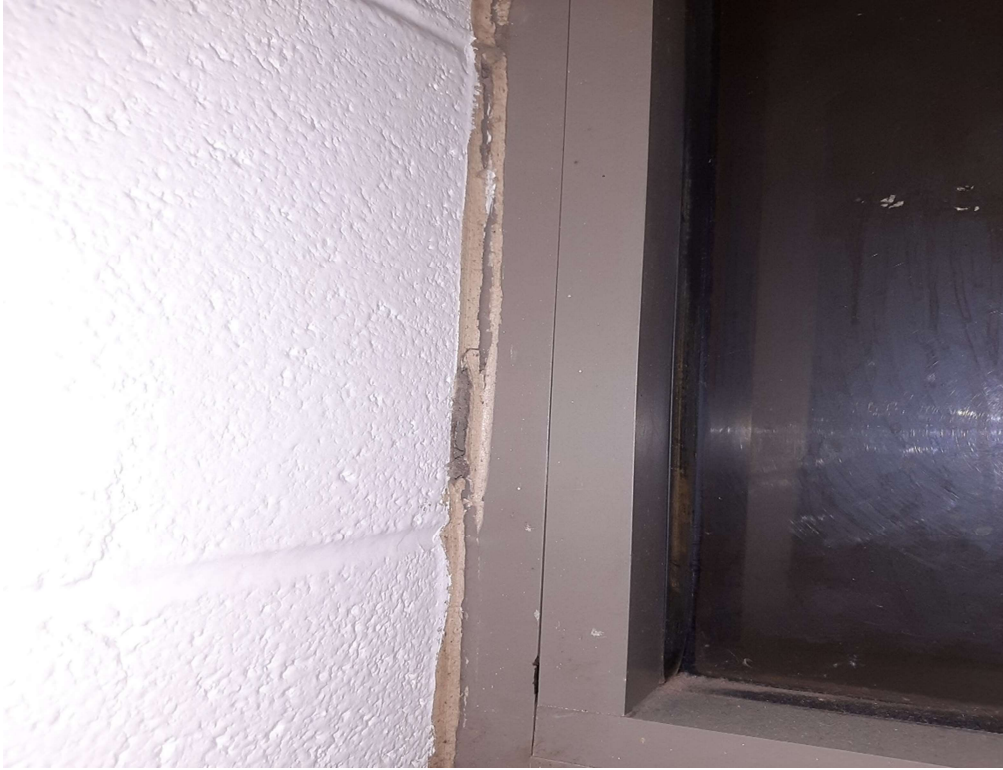
Photograph No. 9 – Hard beige interior sealant on the 2 nd floor hallway window contains asbestos.
