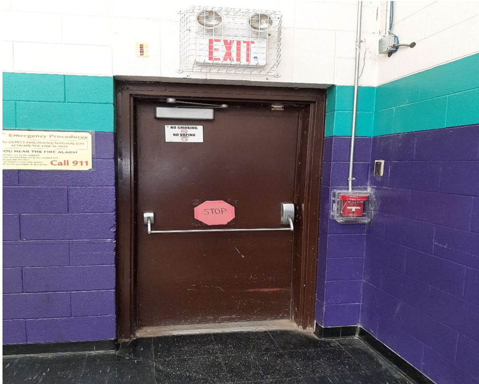
Photograph No. 8 – Black vinyl floor tiles around the exterior door in the gym contain asbestos.
