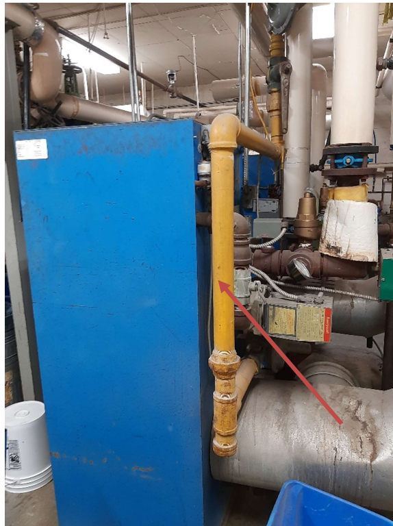
Photograph No. 4 – Yellow paint on the gas lines was sampled (LP03) and is lead-based.
