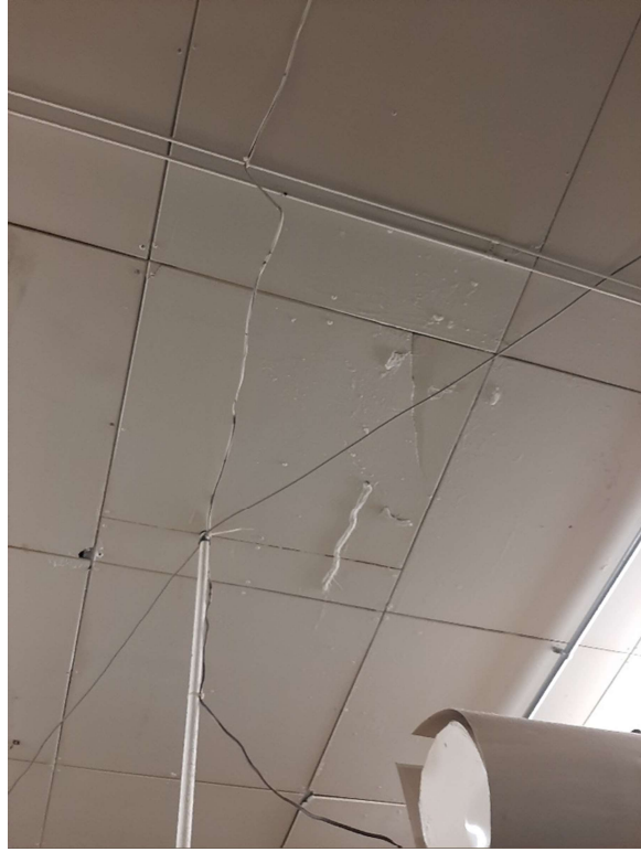
Photograph No. 1 – Asbestos-containing cement (Transite) ceiling panels are present within the boiler room.
