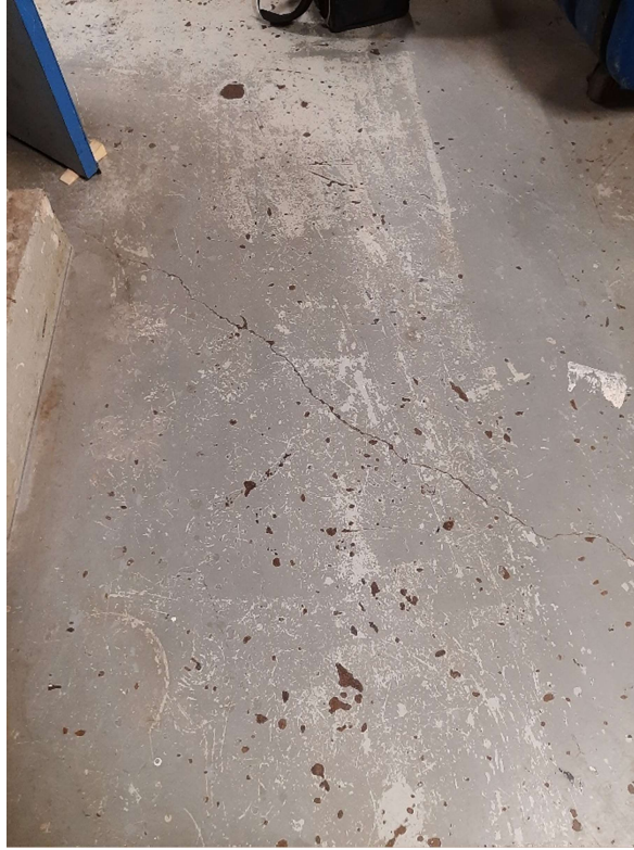
Photograph No. 5 – The grey paint on the floor of the boiler room was sampled (LP02) and is lead-containing.
