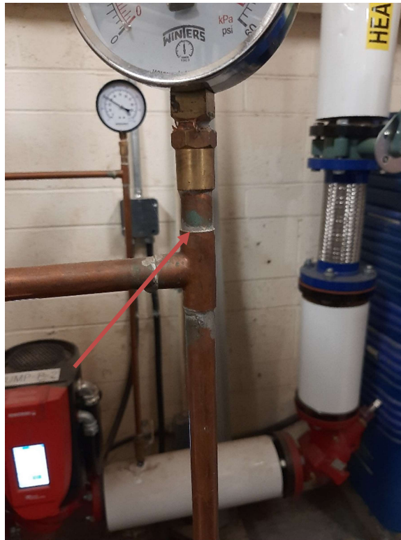
Photograph No. 3 – Suspect lead-containing solder on copper pipe connections was observed within the boiler room.
