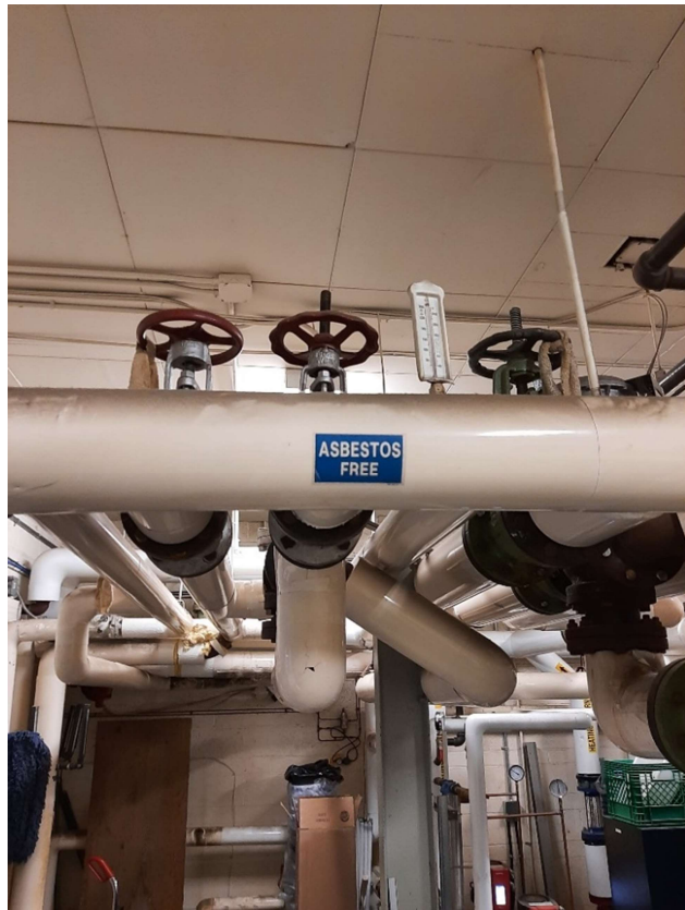
Photograph No. 2 – Pipe straights and elbows consist of PVC over fiberglass and are not suspected of containing asbestos.
