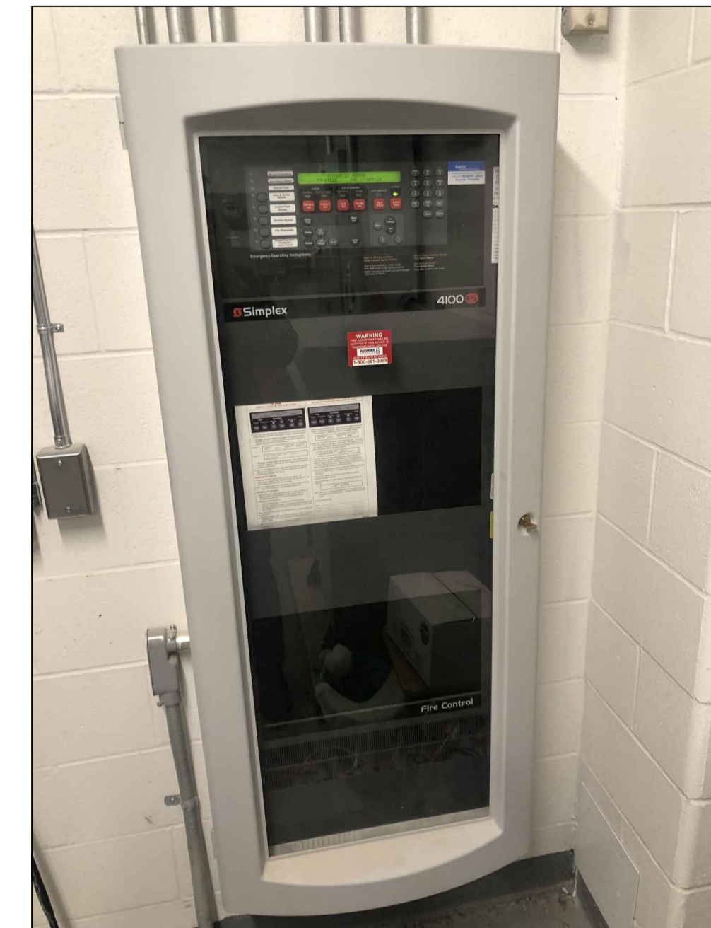
PHOTO – MAIN FIRE ALARM CONTROL PANEL (SIMPLEX 4100 ES)
