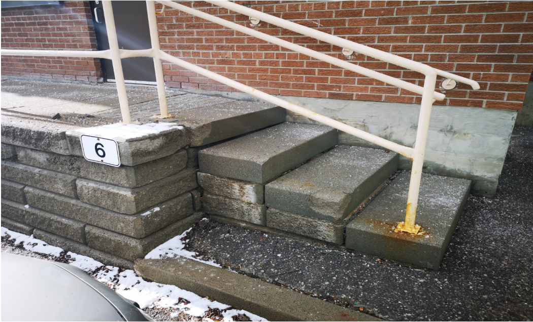
Fig. # 9 View of steps. Note deteriorated guard rail.
