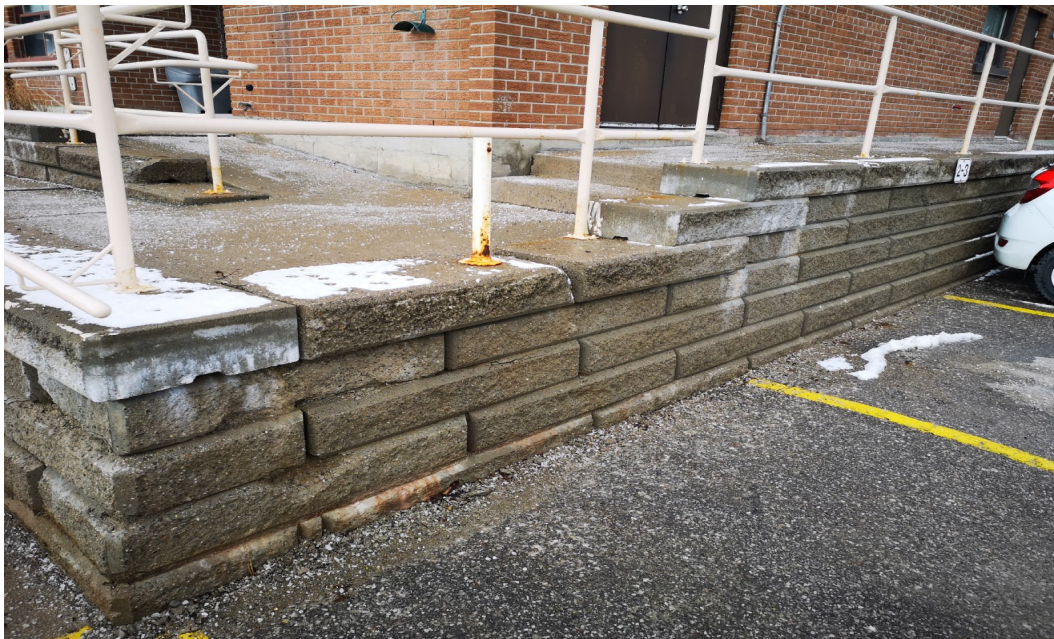
Fig. #4 Another view of deteriorated retaining wall.
