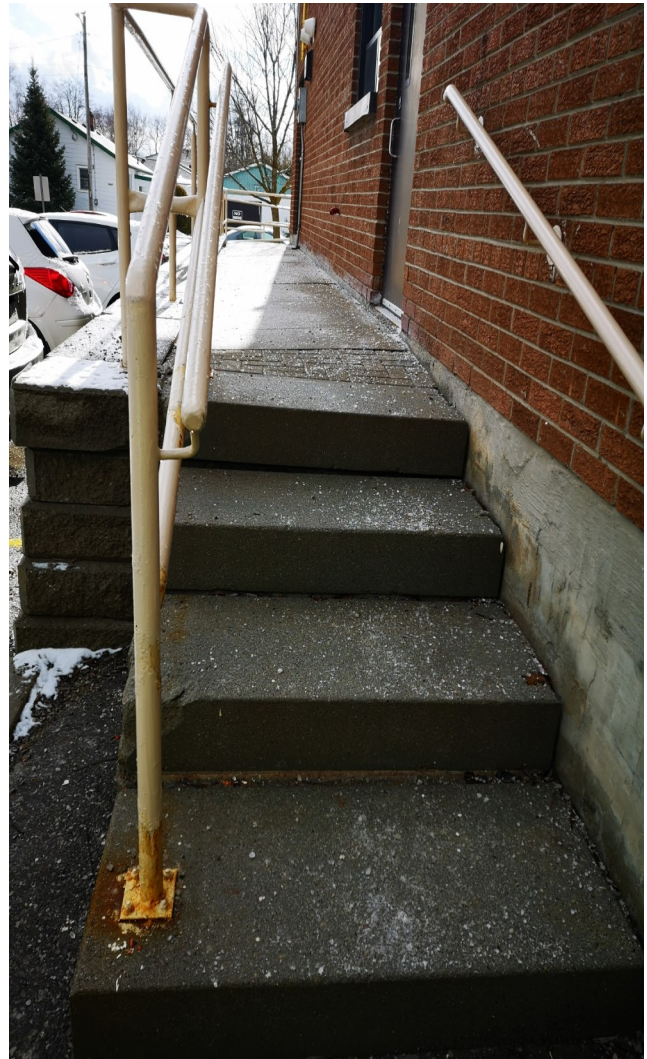
Fig. #8 Side retaining walkway and the steps. Note leaning concrete steps and corroded guard rail base.
