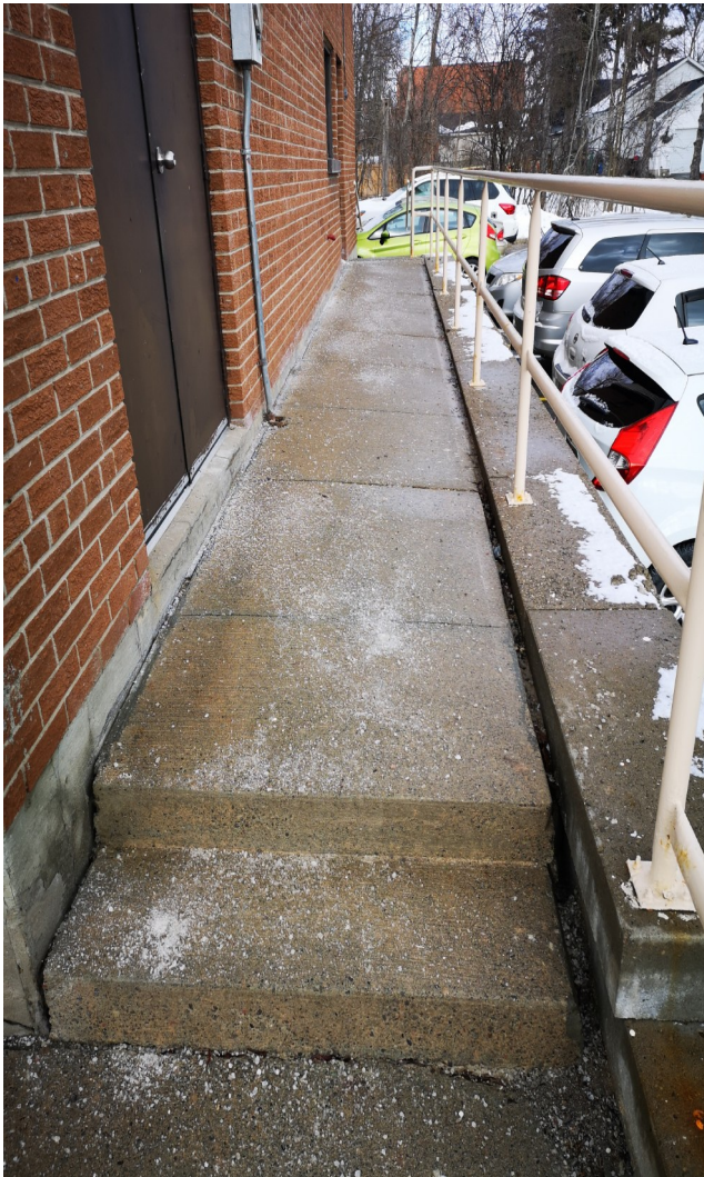
Fig. #7 Side retaining wall supporting walkway. Note leaning concrete.
