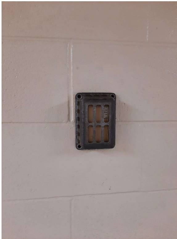
Photograph No. 8 – Mercury containing thermostats were observed in the second floor corridor.
