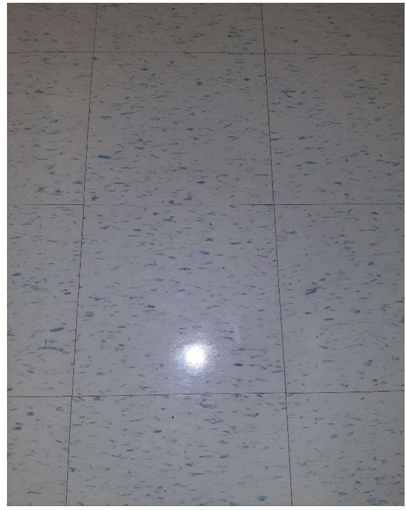
Photograph No. 2 – 12”x12” White with blue fleck vinyl floor tiles observed in Room 167 were sampled (S01A,B,C). The tiles and mastic are non-asbestos.
