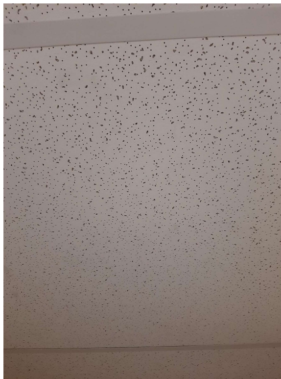
Photograph No. 4 – 2'x4' small fissure random pinhole ceiling tiles were observed in room 102 and were sampled (S04A,B,C). The ceiling tiles are not asbestos-containing.
