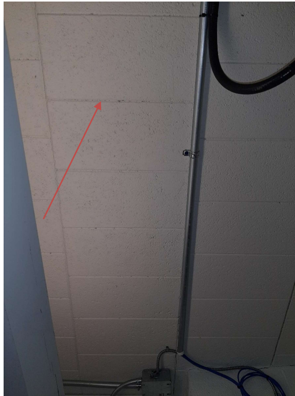
Photograph No. 3 – The concrete mortar on the ceiling of room 167 was sampled (S02A,B,C) and is not asbestos-containing.
